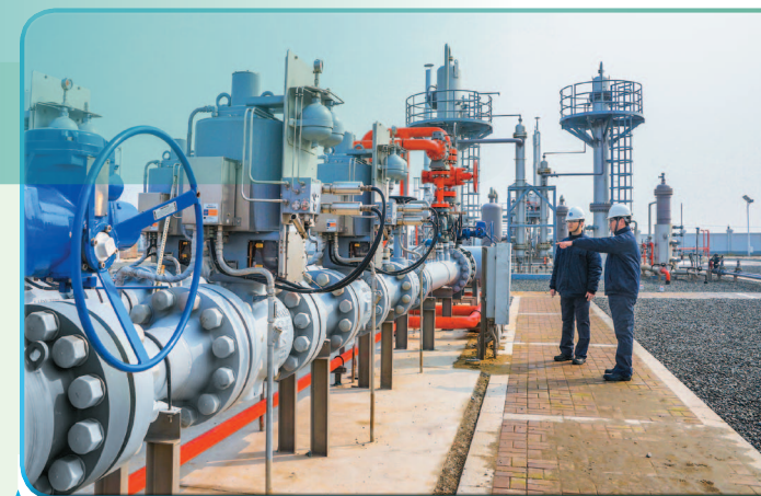
The Group’s underground gas storage facility in Jintan District, Jiangsu Province, provides emergency peak-shaving reserves for the country.
